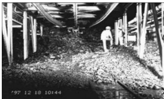
Photo 1. TBM Deeply Buried by Large Amounts of Debris after Inundation.
